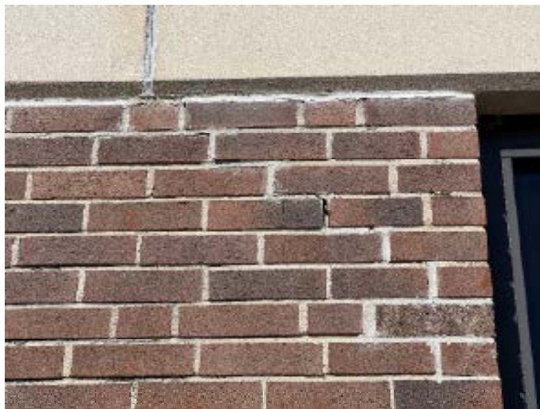
Figure 3 – Diagonal Crack Building on Brick Veneer
