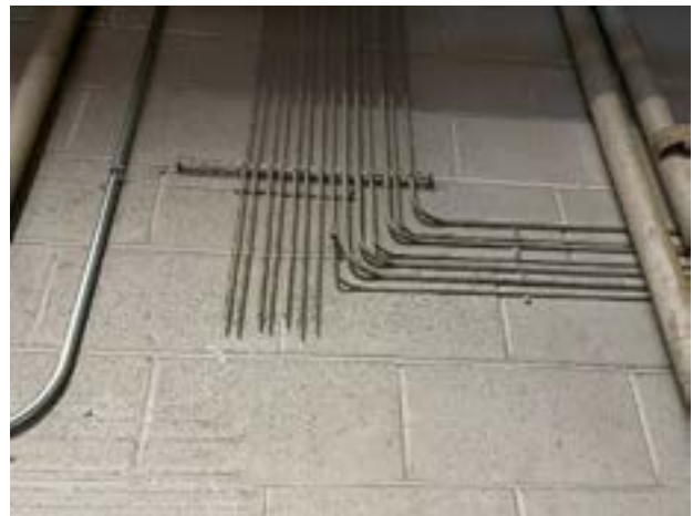
Abandoned/Cut Pneumatic Control Lines
