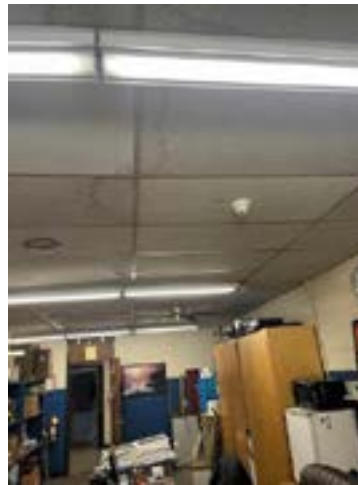
Fixtures Missing Lens
