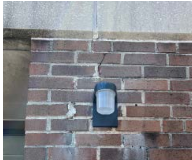
Figure 2 – Crack in Brick Veneer
