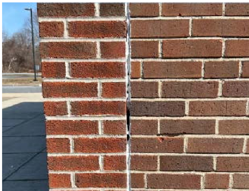
Figure 5 – Missing caulking at a Wall Joint
