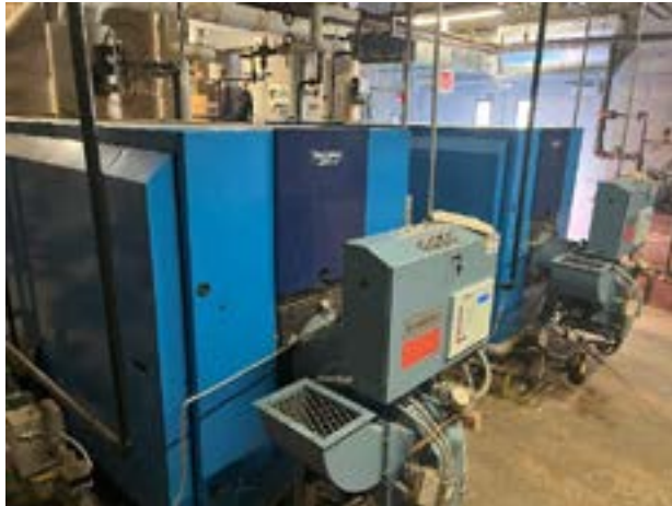
Existing Steam Boiler Plant
