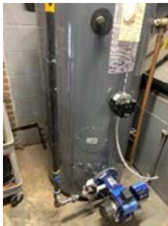
Gas Water Heater
