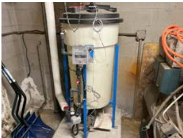
Glycol Make-up System
