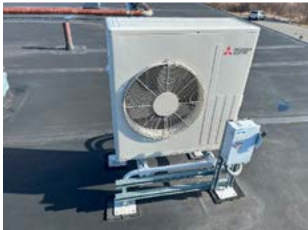
Typical Outdoor Terminal of Split Unit
