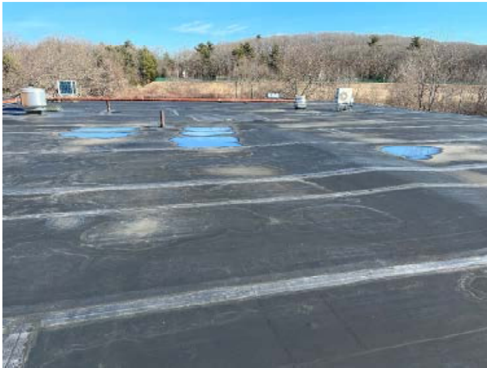
Figure 7 – Water Puddles on Roof
