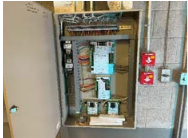
Controllers within Control Cabinet
