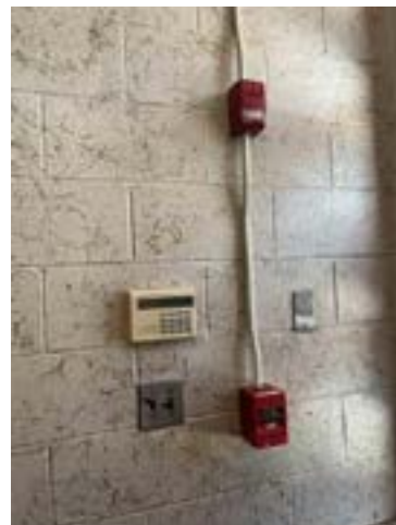
Pull Station/Horn Strobes
