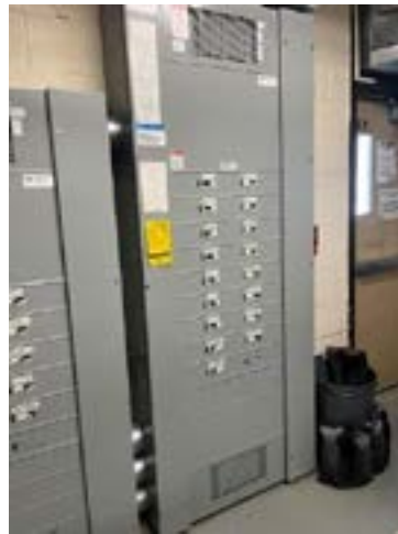
"MDP" Main Distribution Panel
