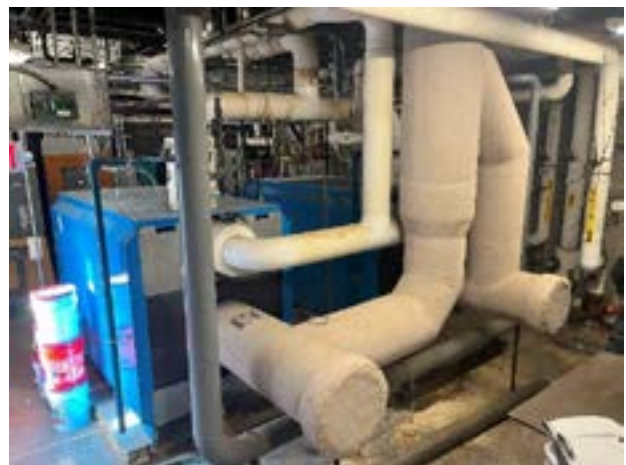
Insulated Boiler Venting to Chimney
