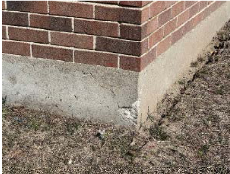
Figure 4 – Diagonal Crack in Foundation Wall Corner.
