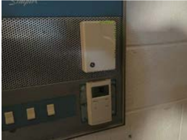
Typical Room DDC Sensors
