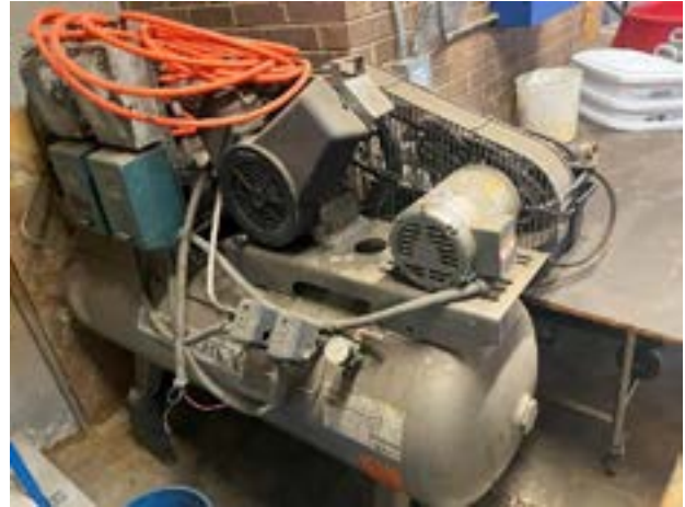
Abandoned Pneumatic Control Compressor
