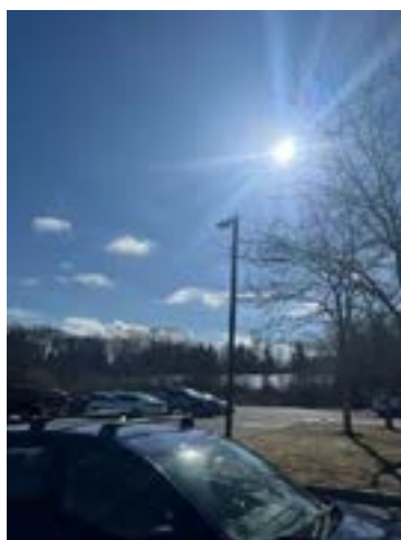
Site Area Light Fixture
