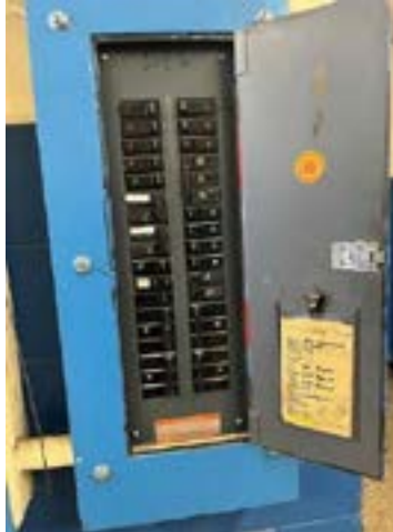
Original Vintage Panelboard
