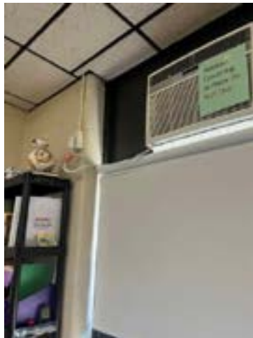
Receptacle for Window A/C
