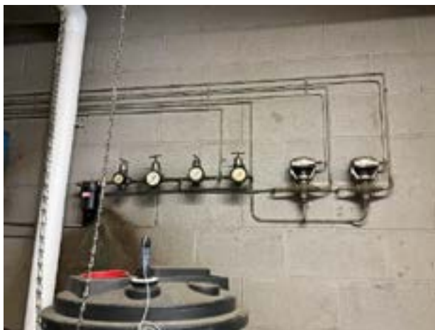
Abandoned Pneumatic Control System Gauges
