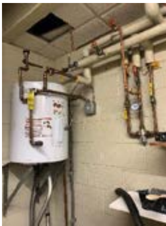
Electric Water Heater
