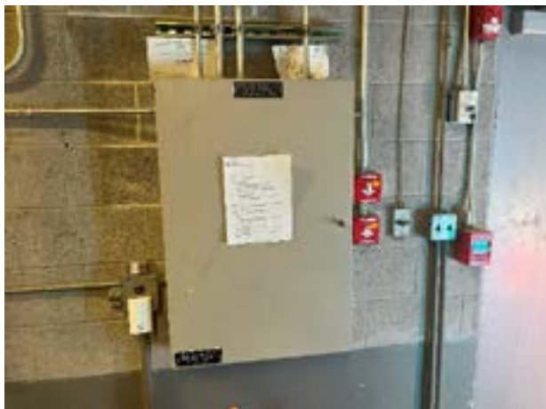
HHW Plant Control Panel
