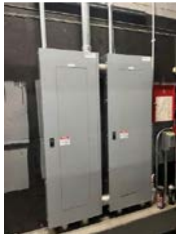
2011 Vintage Mechanical Panelboards
