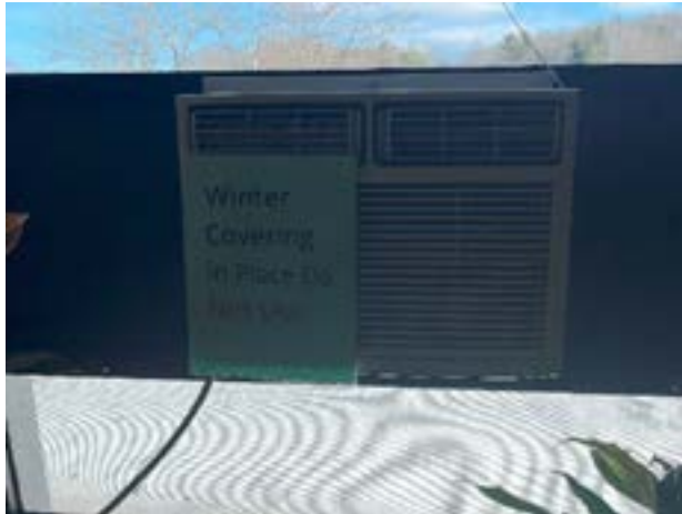
Typical Window Air Conditioner
