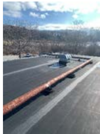
Gas on Roof
