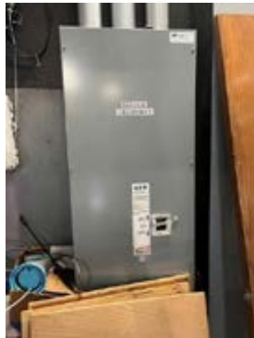
Main Service Disconnect
