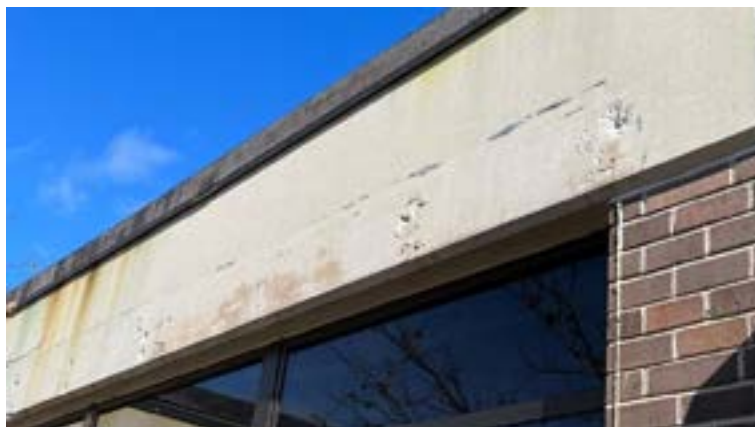
Figure 1 – Spalls in Precast Band Beam
