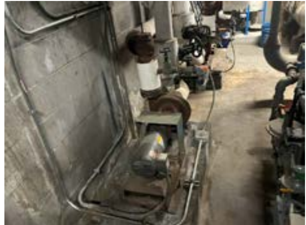
Typical Hot Water Pumps
