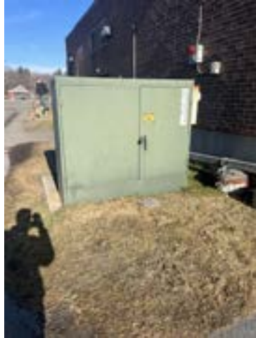
Pad Mounted Transformer
