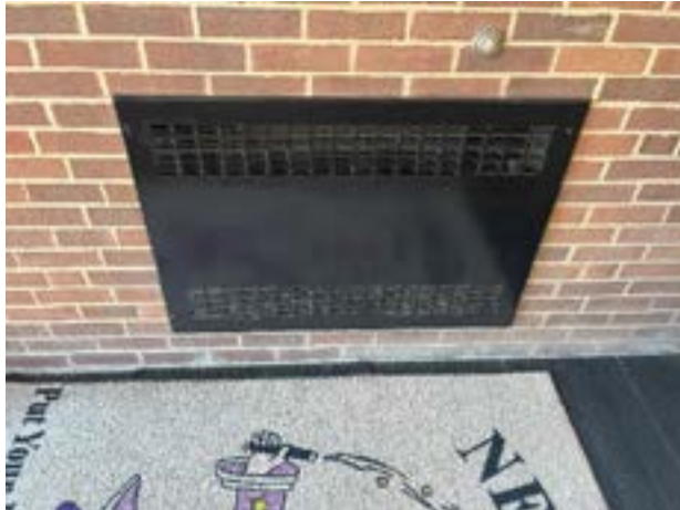
Typical Hot Water Convactor
