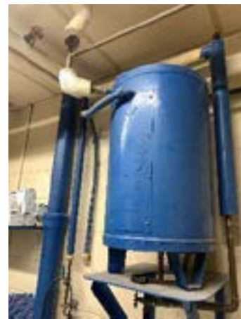
Electric Water Heater
